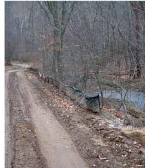
Encroachment on SMZ with silt fence for control
